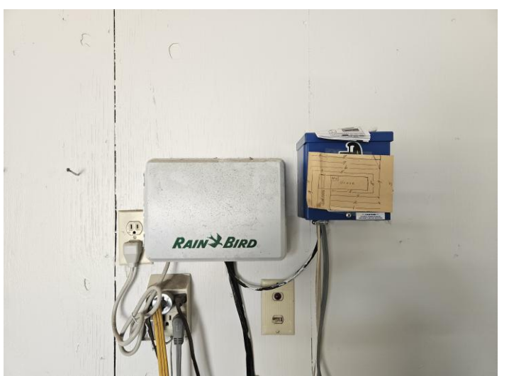
Underground Sprinkler control box
