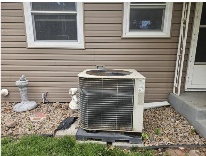
Central Air Unit
