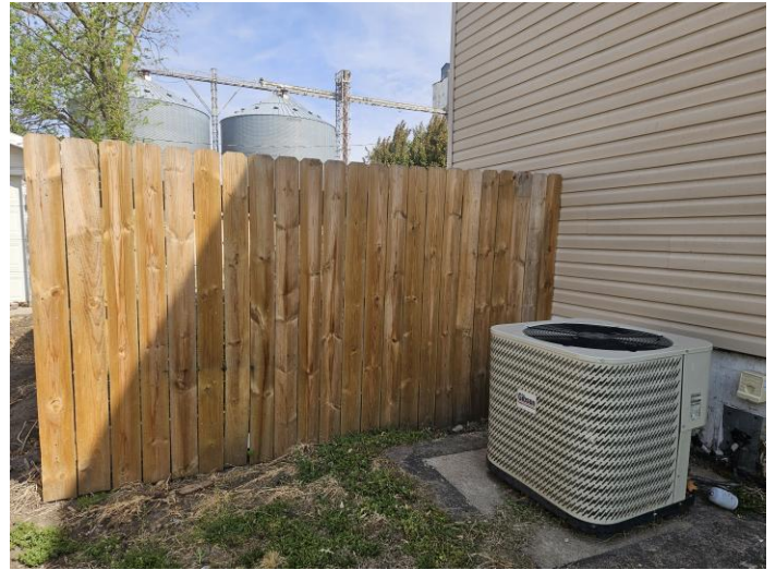
New Wood Fence and Central Air Unit
