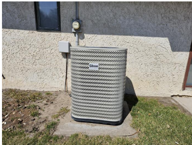
Central Air Unit
