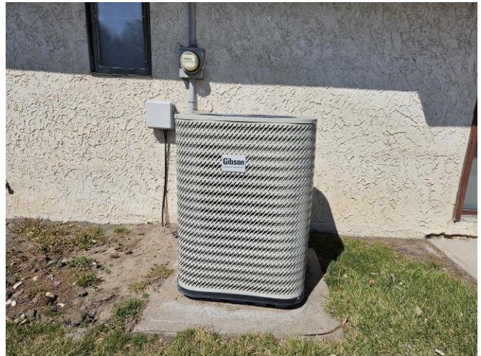
Central Air Unit
