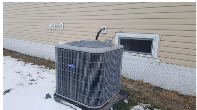
New carrier air conditioner unit
