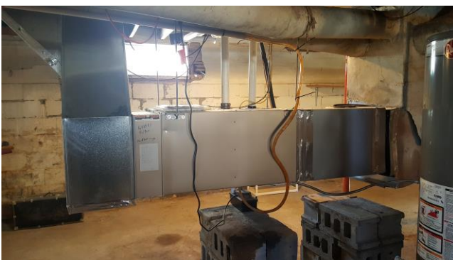
New Carrier Furnace
