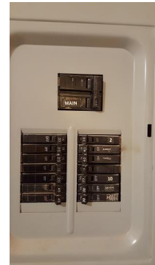
circuit breaker box
