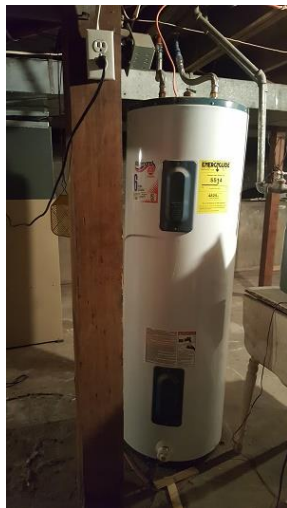
New hot water heater
