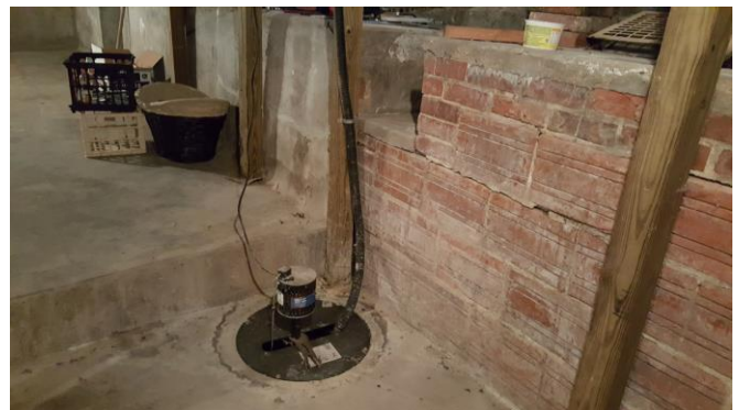
New sump pump
