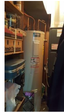
Hot Water Heater
