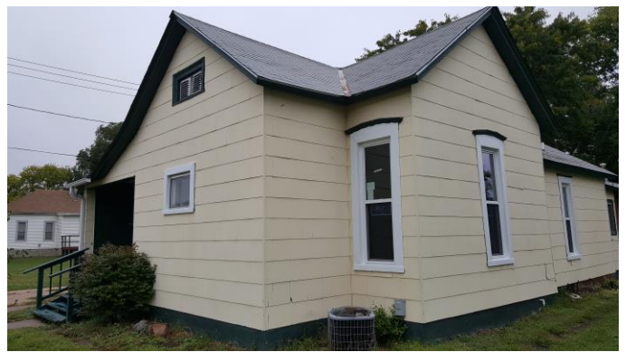
South side & central air unit
