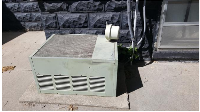
Central air unit
