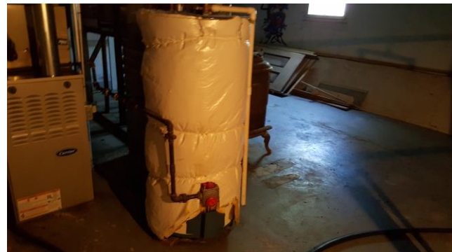
Hot Water Heater
