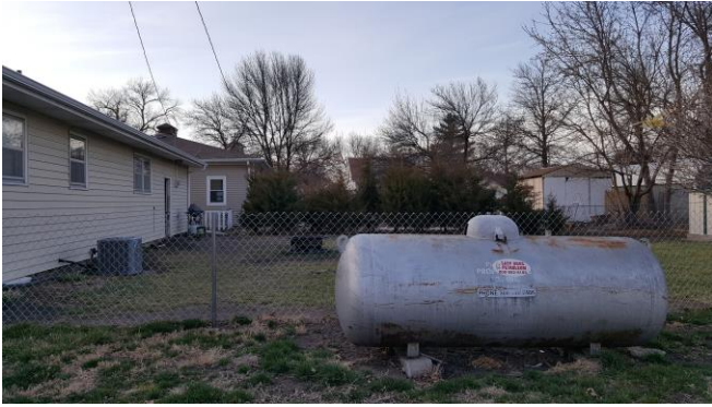
Rented Propane tank
