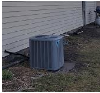
New Central Air unit
