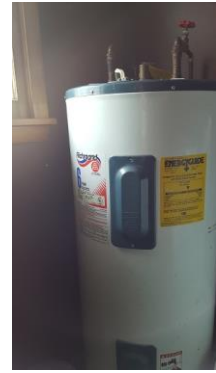
Hot water heater
